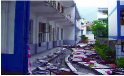
图8 无拉结筋的女儿墙、栏杆塌落(通济学校) Fig. 8 Collapse of parapet wall parapet and railing without binding rebar (Tongji Middle School)
