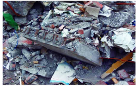
图10 板侧无灌缝咬合整体性差而坠落(聚源中学) Fig. 10 Falling board without irrigation side seams (Juyuan Middle School)
