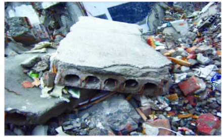
图11 预制板端无连接锚固措施而坠落(聚源中学) Fig. 11 Falling board without connection anchorage measures at block ends (Juyuan Middle School)
